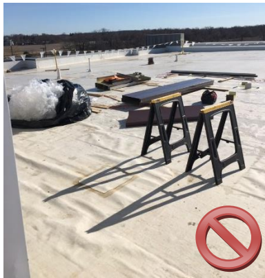
Roof Damage caused by lack of protection
