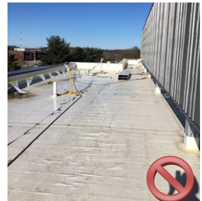
Roof Damage caused by lack of protection
